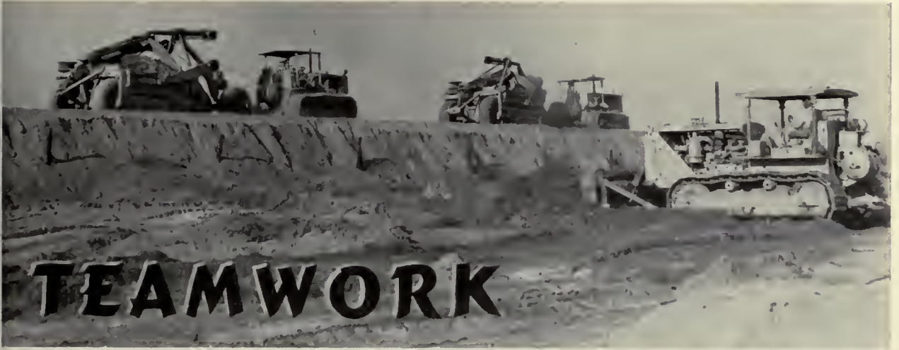
BUILDING UP THE LEVEES. —All photos for this article by Herbert Huffman, San Joaquin Valley District.
